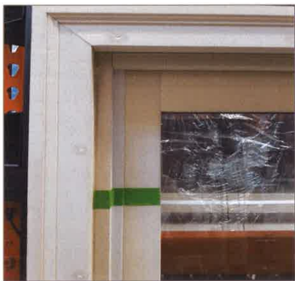
Figure 1: Reveal measurement is indicated by tape in the following photo (inside edge of exterior trim to the point where the glass surface begins).
